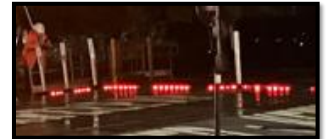
Delineators & Solar Markers @ night.
