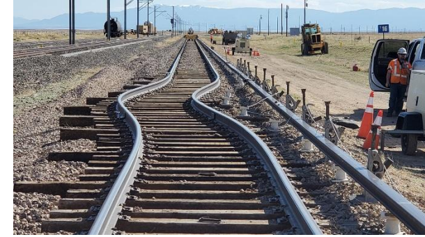
Example of track damage
