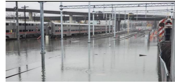
4 th & King Flooded Track January 2023
