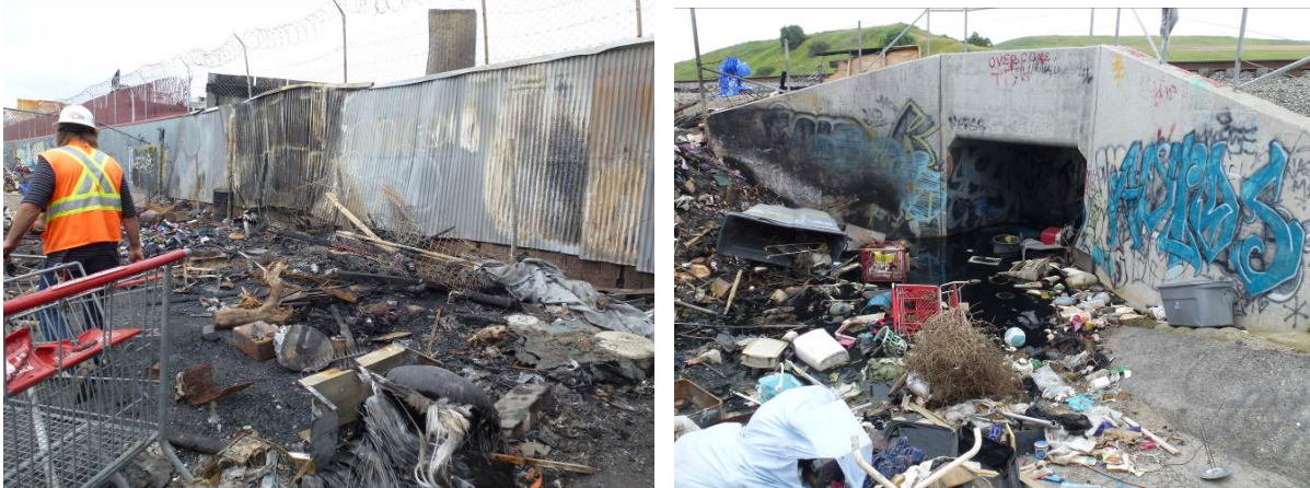
Post Fire Debris
