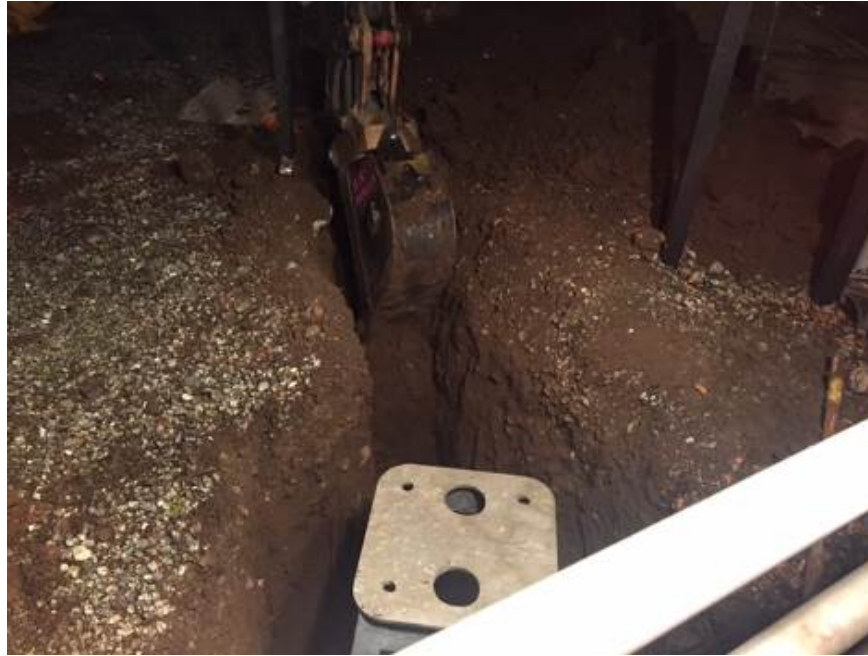
This work was in preparation for upcoming improvements at Ravenswood Avenue grade crossing in Menlo Park
