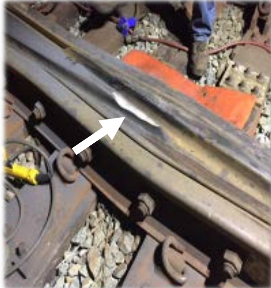
Metal flaws are removed
