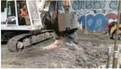
Subsurface conditions more difficult than expected
