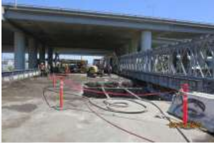
Existing concrete deck thicker than expected
