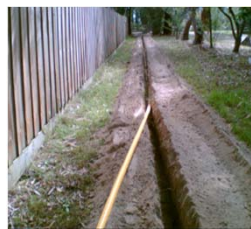
Conduit placed in trench (~42" deep x 9.5" wide, within the Caltrain right of way)
