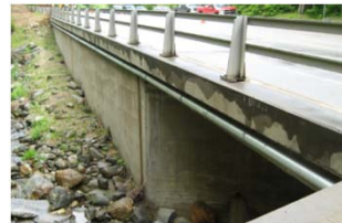
Conduit on tunnel or bridge (clamps/hangers, may require lane closure during off-peak hours)
