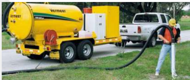
Potholing (Vacuum-excavation preparing the job site, within the Caltrain right of way)
