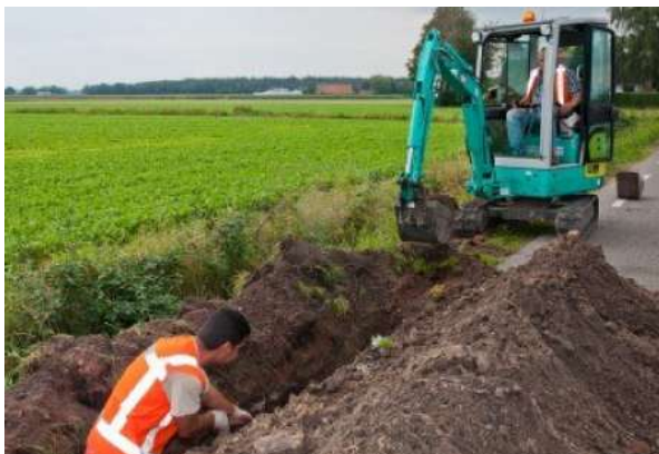
Trench (with mini excavator or by hand, within the Caltrain right of way)
