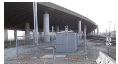
Base Station Hut in the Right-of-Way
